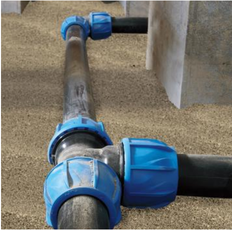
Water Distribution Lines
